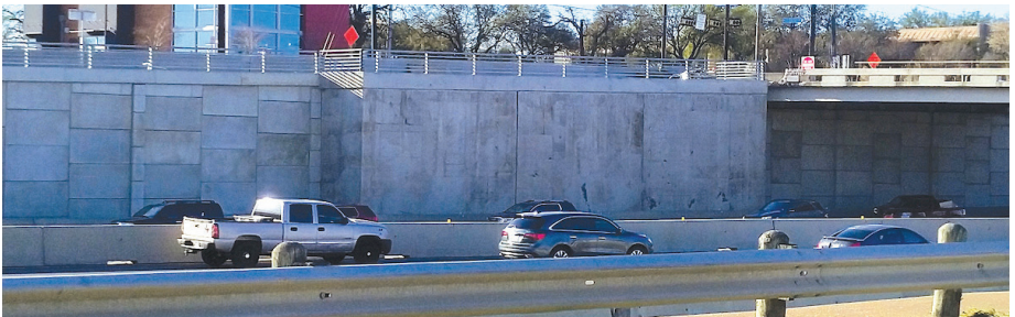
Highlighting the revised design (extended portion) of the retaining wall on TX 360 north of IH 30. This portion of the retaining wall was extended due to a change in the foundation design to mitigate a conflict with a utility duct bank.
